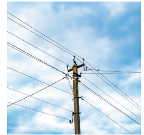
Electrical and Utility
